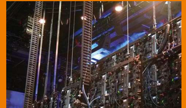
Vertical energy supply systems for theatre and stage technology
