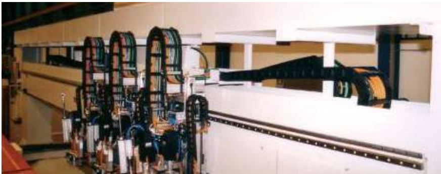
Woodworking machines with e-chains® and chainflex® cables
