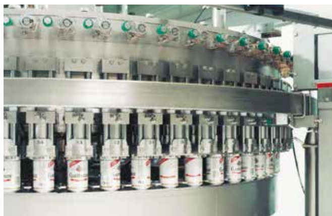
Filling machine, Kronen AG, Rosenheim (Germany)
